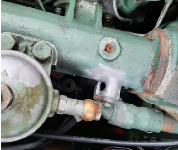
The narrowboat owner noticed the 15mm x 15mm hole in the engine heat exchanger manifold whilst moored on a canal 30 miles from London
