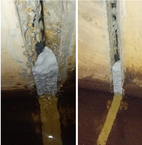
The original sealing compound between concrete slabs had washed out of the flood defence wall, with the resulting gaps packed with AB Original
