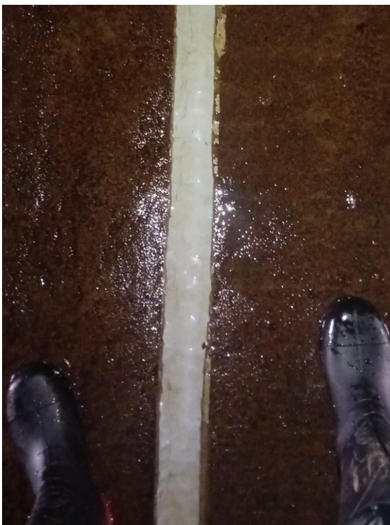
Gaps in the concrete floor submerged by flood water were also sealed thanks to the underwater curing properties of AB Original
