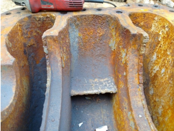
The pump housing was heavily damaged by years of extracting water containing silt, sand and other debris
