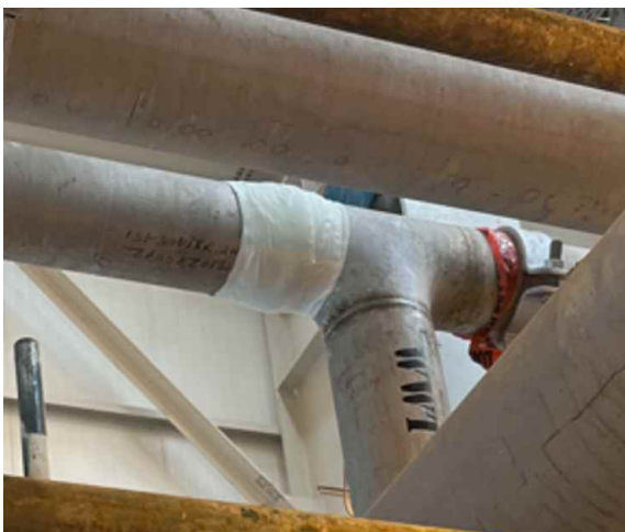
Repairs were reinforced with SylWrap Bandage - and were made to difficult sections of overhead pipe
