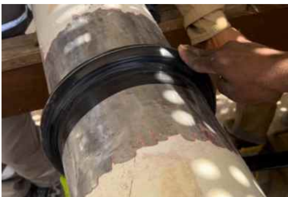
Multiple Wrap & Seal applied to leaking welding joints built repairs capable of holding 10 bar pressure
