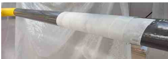
SylWrap increased the thickness of the weakened area where the pipe had contact with the U-support
