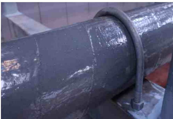
A second Liquid Metal coating was applied over the SylWrap and the pipe fixed to the U-support
