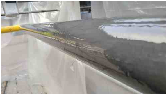
Rust, grime and paint were ground off the pipe and the three metre section coated in Liquid Metal
