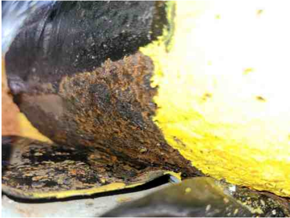
The pipe was heavily corroded where water had been trapped between a protective PVC tape and the line
