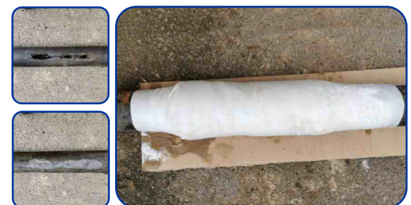
When pressure can be stopped, epoxy putty fills in holes, cracks and missing sections
