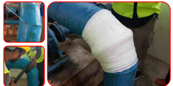
When pressure cannot be stopped, pipe burst tape is wrapped tightly around the leak area
