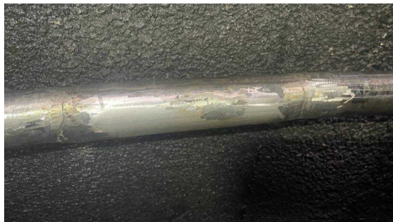
An initial repair attempt involving patch welding failed, leaving multiple pinhole leaks in the pipe
