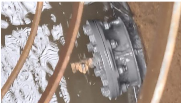
The stub needing encapsulation was difficult to access at the bottom of a chamber surrounded by metalwork
