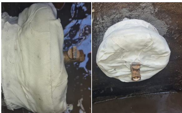
SylWrap HD was wrapped around the stub and smothered over the flange plate for protection
