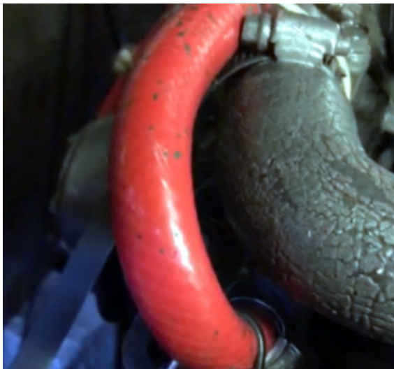
The pinhole was on a section of red coloured rubber pipe where access was severely restricted
