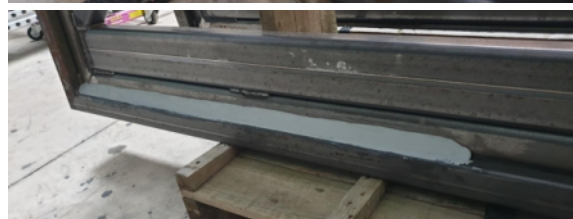
Putty formed into a bevelled edge to prevent water gathering at the base of the frame
