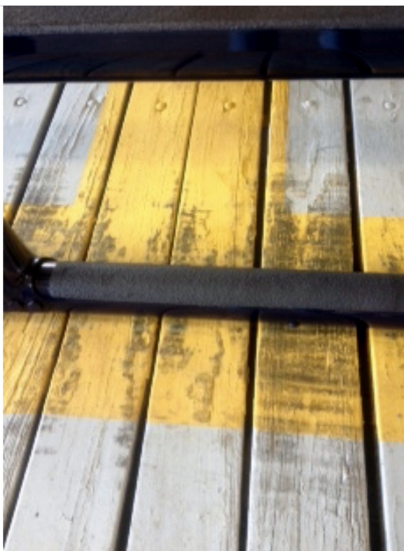
Liquid Metal was coated onto the legs and silicon carbide deposited over the top. Once the epoxy had cured, the grit was permanently bonded to the skids to create a long term anti slip solution
