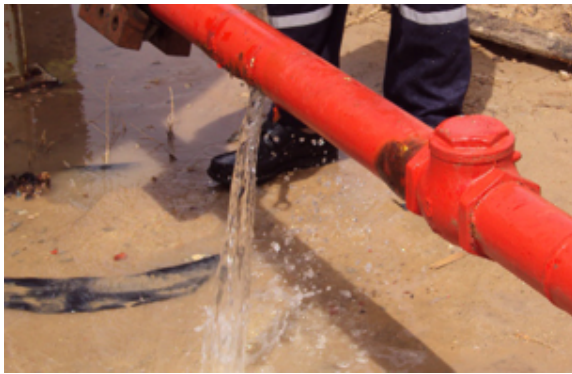
Significant levels of water were escaping the above-ground section of pipe at 5 bar pressure from a longitudinal split
