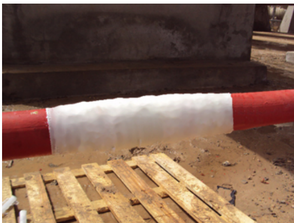
The above-ground section having been successfully repaired using Wrap & Seal and then overwrapped with SylWrap HD
