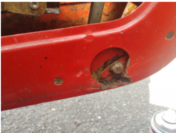
Moisture Repellant Spray was used to drive moisture and grease from the hole before the metalwork was further cleaned via the removal of dirt, grime and rust
