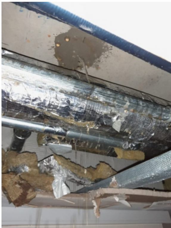
Steel pipe can be seen across the middle of the photo, spraying water which was damaging surfaces
