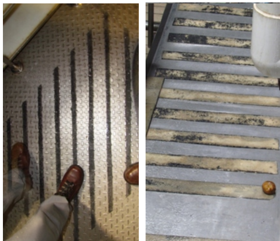
Existing anti slip surfaces at the plant needed to be replaced having become worn and ineffective
