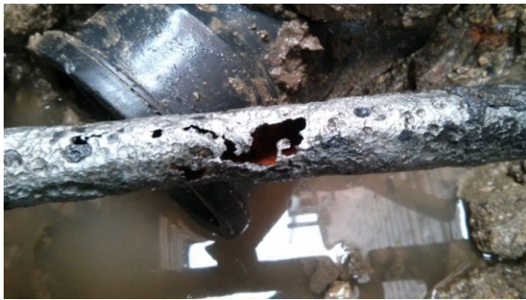
The larger crack in the malleable iron water supply pipe and several smaller holes surrounding the damage area
