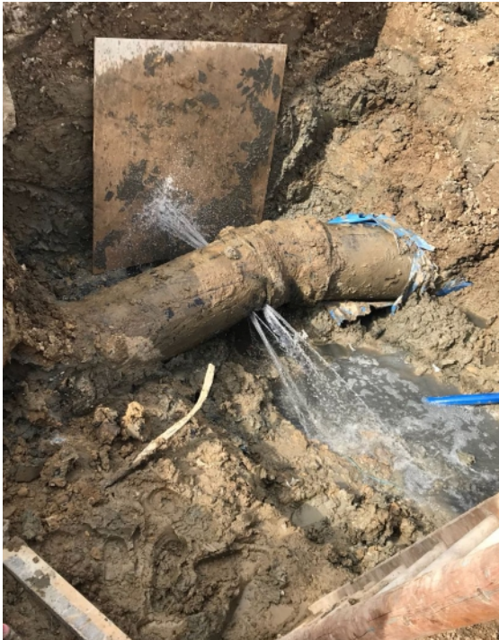
Significant amounts of contaminated water were escaping from the damaged pipe
