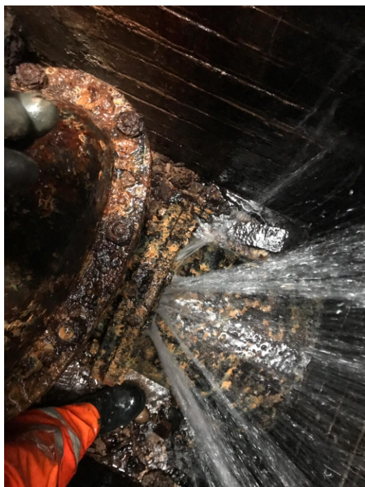
The split in the 400mm carbon steel water main possessed a significant challenge
