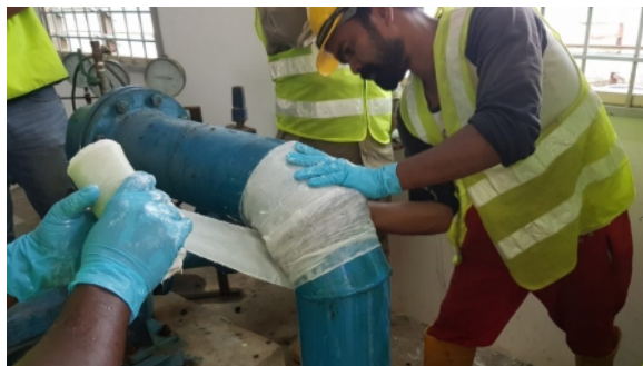
SylWrap HD reinforced the initial repair, smoothed around the pipe to create a protective sleeve
