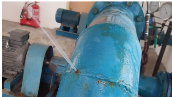
A jet of water was escaping the elbow at 6 bar from a pinhole leak caused by corrosion
