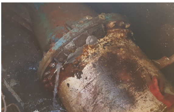
A valve was fixed in place with epoxy to channel water escaping through a gap between flange and pipe
