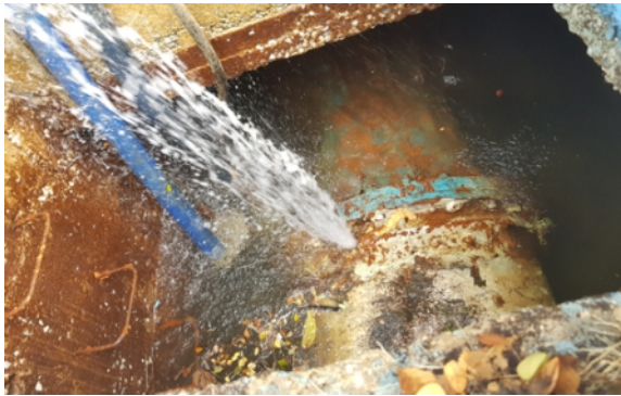
Pressurised water spraying from cracks in the main as the flooded chamber was drained before repair
