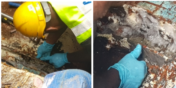
Superfast Steel filled the cracks in the pipe, fixed the plastic plugs in place and encompassed the flange
