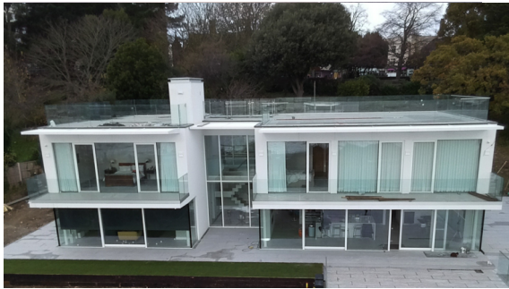
The expansion joints were located between the glass panels on the roof terrace with water dripping through and onto the balcony below
