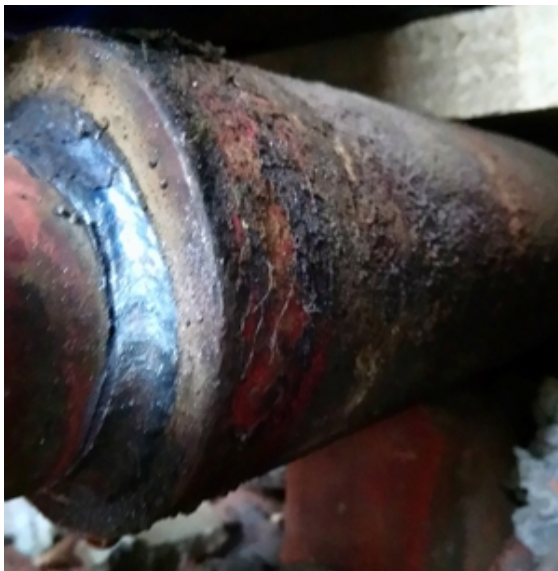
Corrosion to the 100mm pipe at the steel plate
