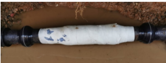
SylWrap HD covered the repair and Wrap & Seal reconnected the cut-out section to the pipe
