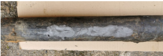
Holes in the pipe sealed with Superfast Steel
