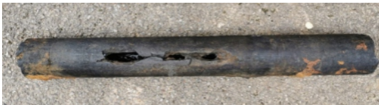
Rupture in the pipe caused by several holes
