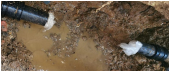
Supply line after the damaged section was cut away
