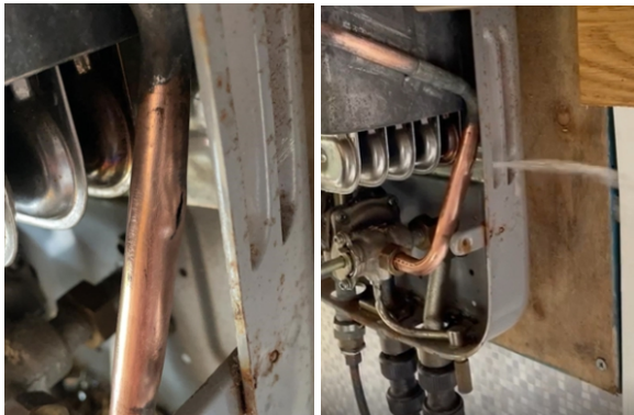
Crack in the pipe was difficult to access. When the boiler system was turned on, a pressurised jet of water sprayed out.
