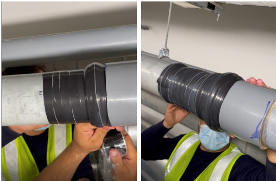
Once the ridge reached level height with the step, wrapping continued to encompass the joint
