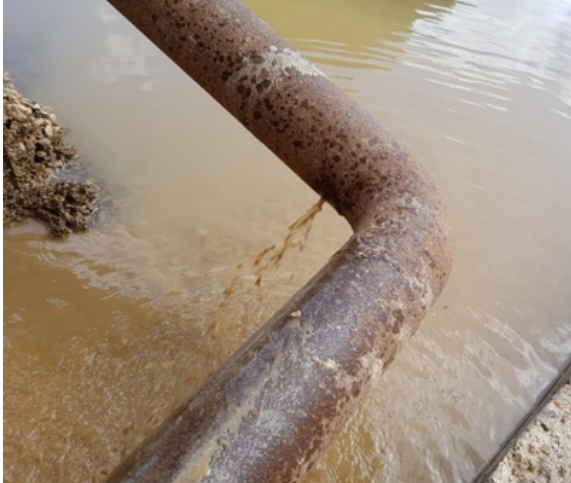
The 150mm steel pipe was leaking from a pinhole close to a 90 degree elbow bend, meaning the quarry could not seal it using their normal method of a pipe repair clamp
